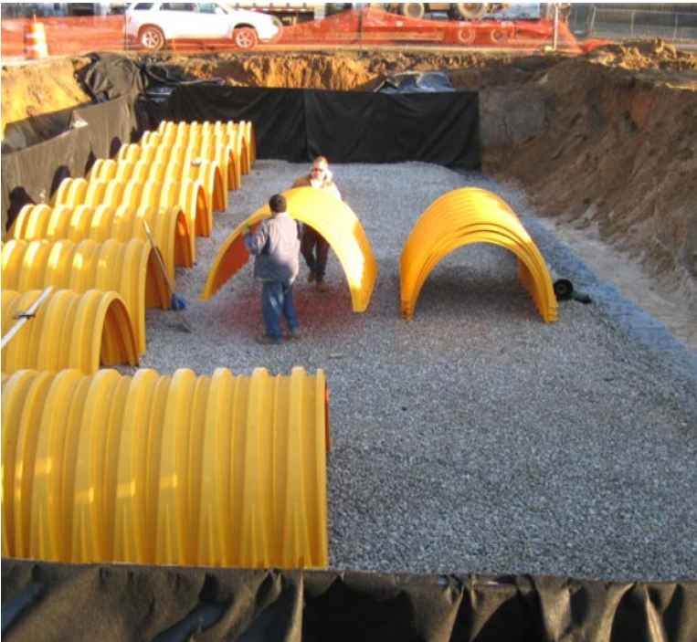
Underground Storage / Infiltration
