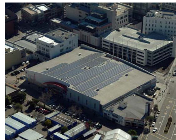
1 MW solar installation on the ice rink downtown
